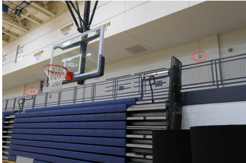
Figure 26: New Mass Notification Annunciators in Gym West
