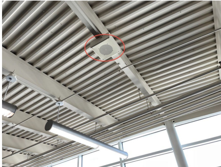
Figure 24: Elevated Ceiling and Speaker in Main Entry Corridor
