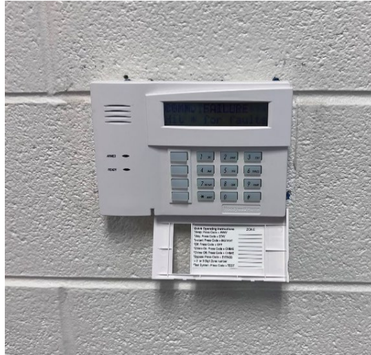
Figure 52: Honeywell Home Alarm Panel with Communication Failure Notice
